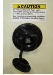
Tank Flush Inlet
