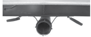
Black/Grey tank drain & valves
